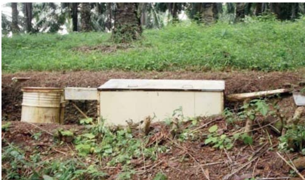
Run off tank with multislot devices
